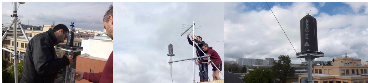
Figure 5 - Installation procedures of the Smart Sound Station, S3 unit, at the campus of ISEL.
