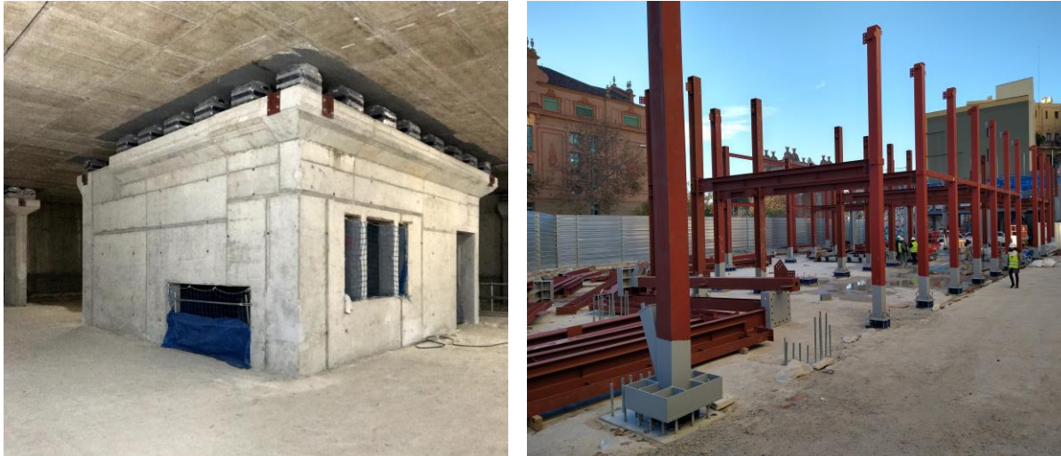
Figure 13. Installation of the Spring isolation in Clinica Girona and Arc de Triomf, respectively.
