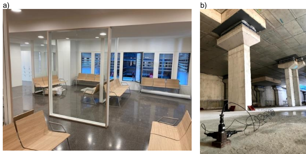
Figure 6. View of some of the measurement points considered for the verification of the building base isolation systems installed in Clinica Girona, a) ground floor and b) first basement floor.
