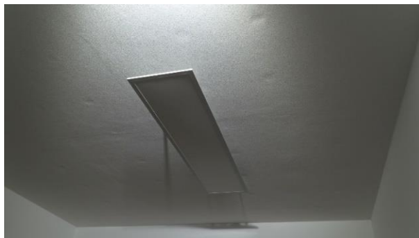
Figure 3 - Seamless ceiling of mineral fibre boards with nonwoven fabric facing, joints and screwing points filled and levelled, sanded, with spray plaster – view in glancing light (photo: Sto)
