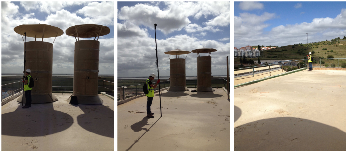
Figure 4 – Example of close field measurement of two noisy chimneys (left) and nearby validation points, in the direction of the residential area.
